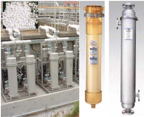
Water purification equipment
